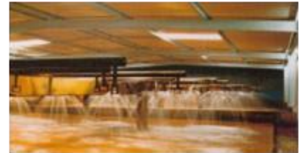
Water extraction and purification
